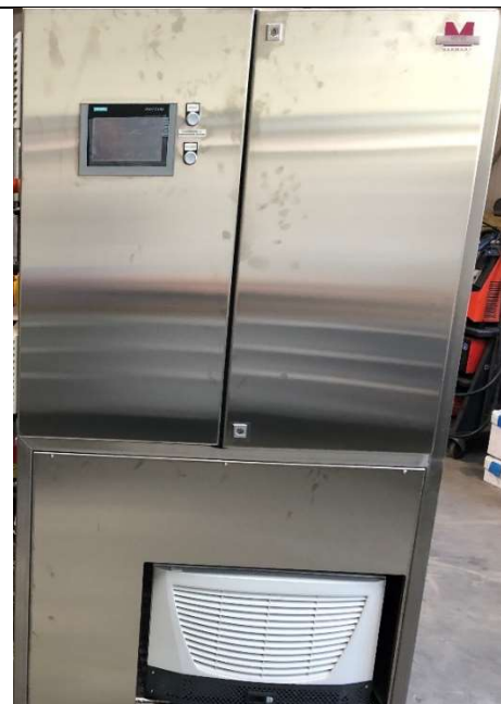
Stainless steel control cabinet
