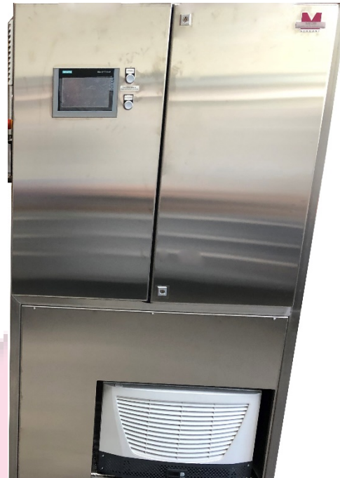
Stainless steel control cabinet
