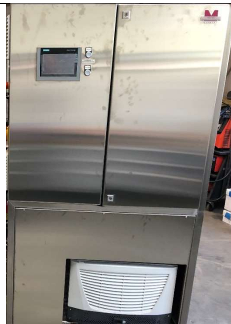
Stainless steel control cabinet
