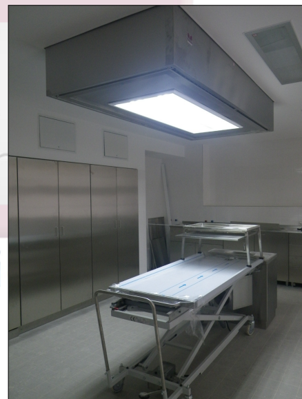
MA-2017 Air supply unit with illumination mounted in intermediate ceiling
