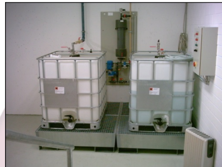
MA-3000 Central Formalin supply and disposal system with 600 litre containers for fresh and waste formalin
