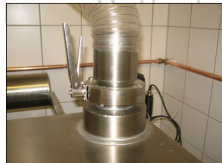
Exit air system via inouse ventilator
